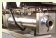
Cooler aluminium protective cladding
